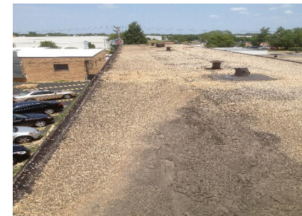
(C) Excessive ponding area
